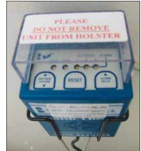
Control unit (CU) secured in wall mounted holster
